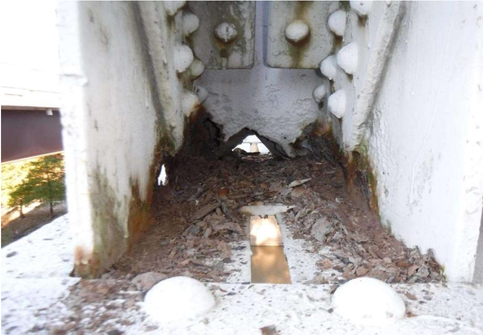
Photo 67 - Lower chord gusset plate condition at Joint L7, Truss 2, Span 5
