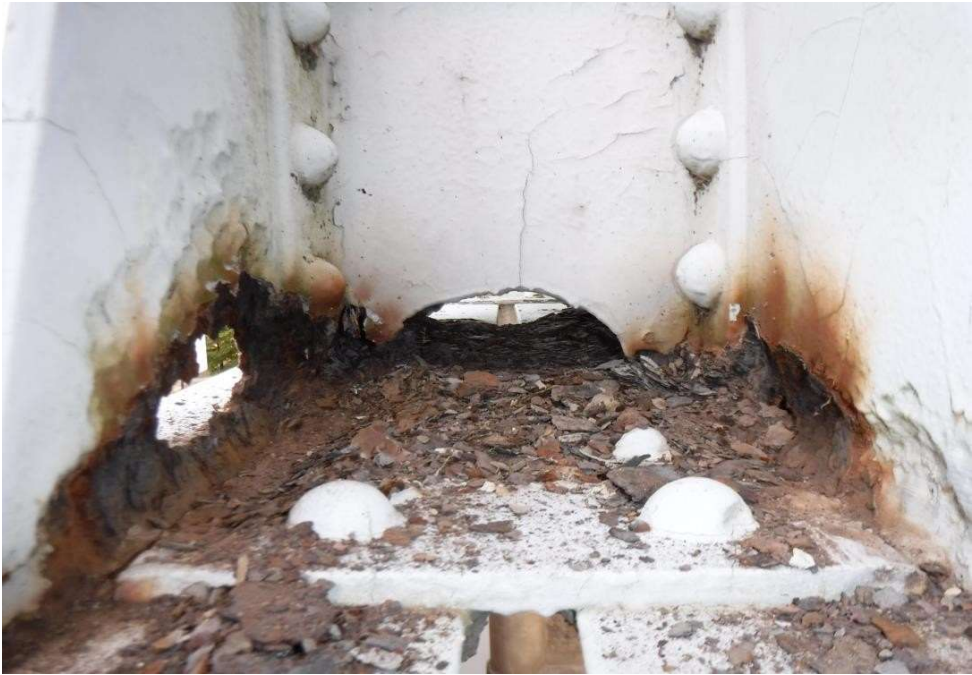
Photo 72 - Lower chord gusset plate condition at Joint L3, Truss 2, Span 6
