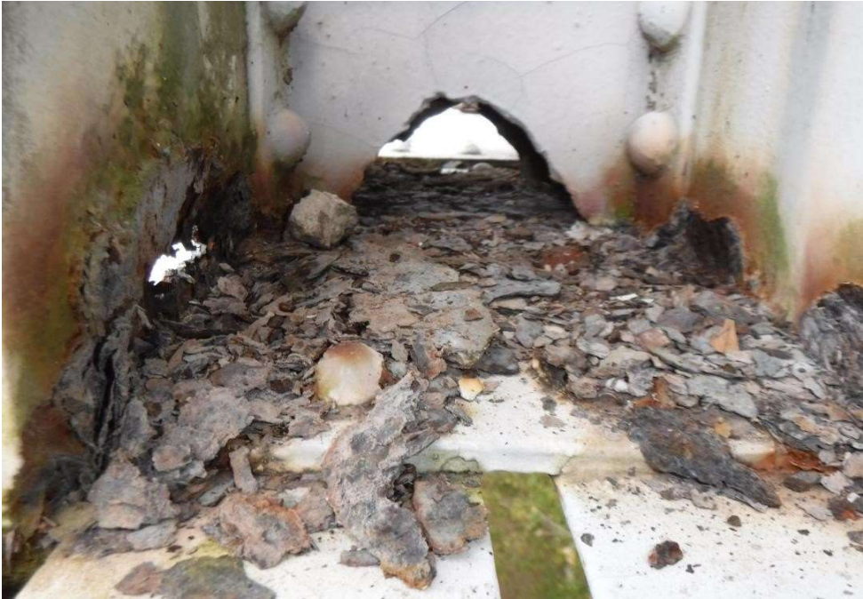
Photo 73 - Lower chord gusset plate condition at Joint L4, Truss 2, Span 6
