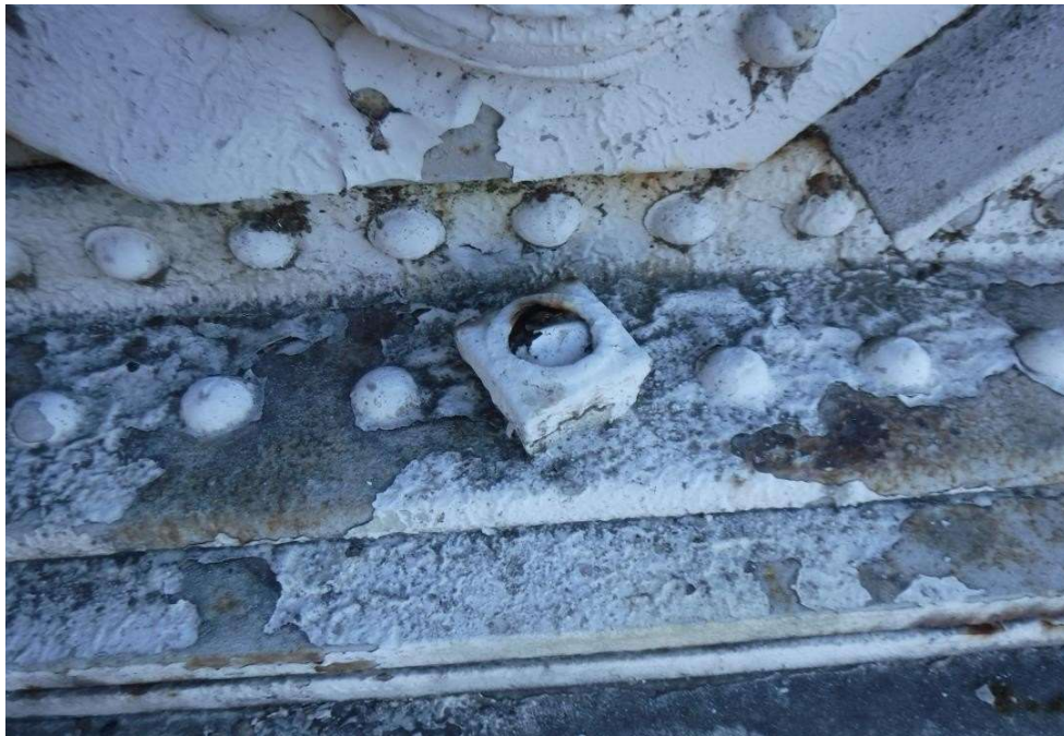
Photo 105 - Exterior anchor bolt condition at Joint L0, Truss 2, Span 5
