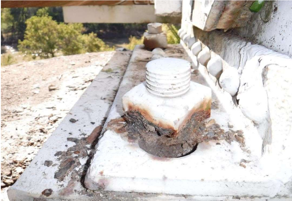
Photo 101 - Exterior anchor bolt condition at Joint L0, Truss 1, Span 4
