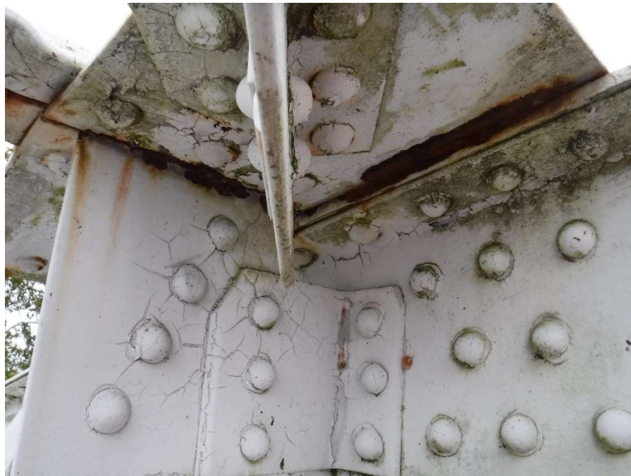
Photo 27 - Typical Section Loss on Horizontal Gusset Plate
