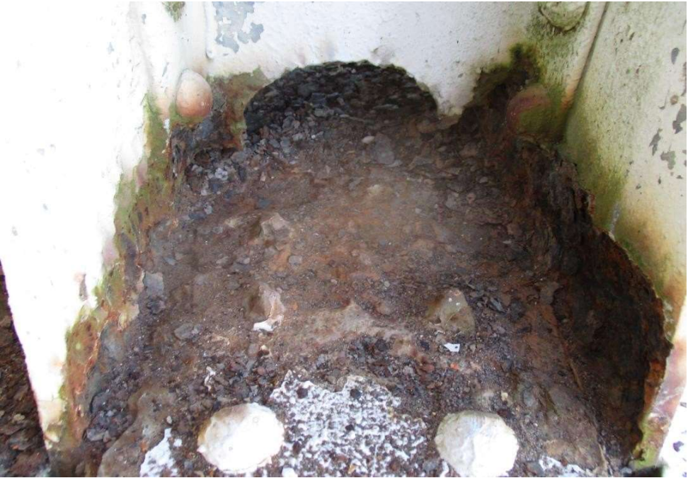
Photo 62 - Lower chord gusset plate condition at Joint L7, Truss 2, Span 4
