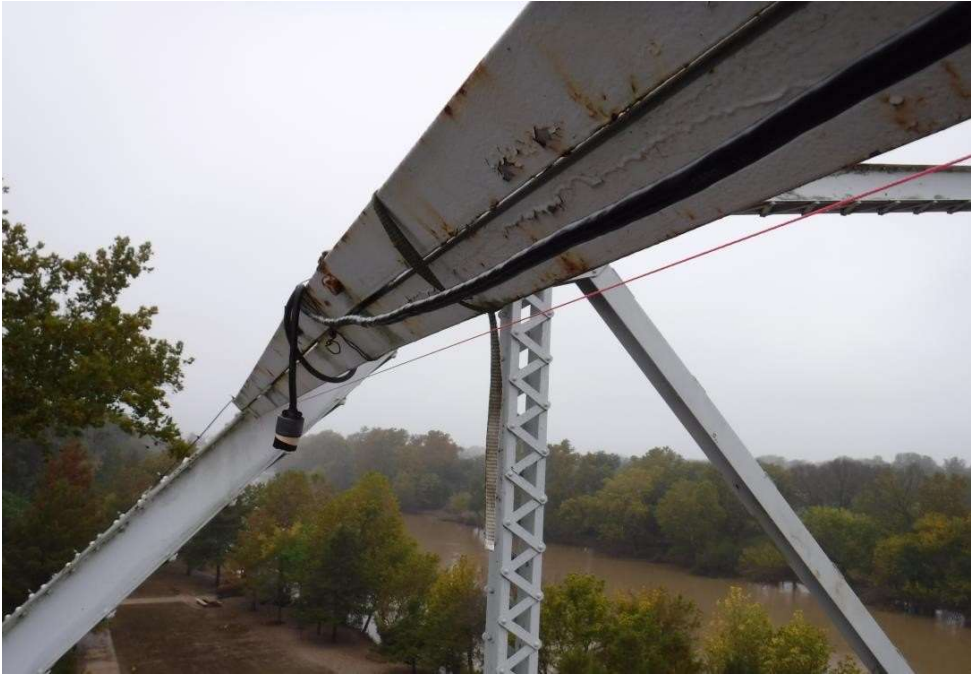
Photo 95 – Cross frame lower chord deformation at Joint U1, Span 4
