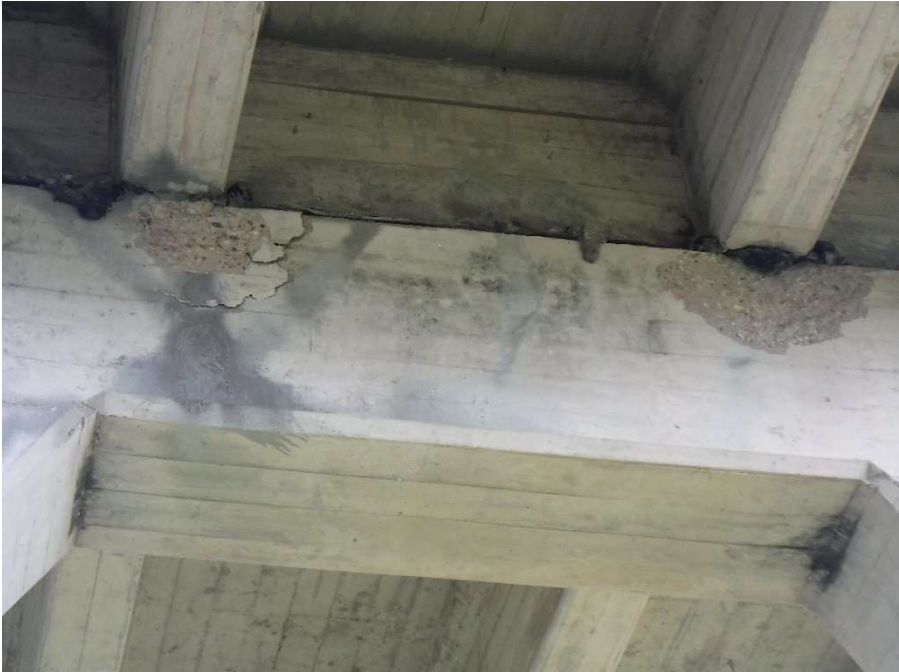
Photo 19 - Delamination and Spalling at Bearing Areas on Bent 13 Cap
