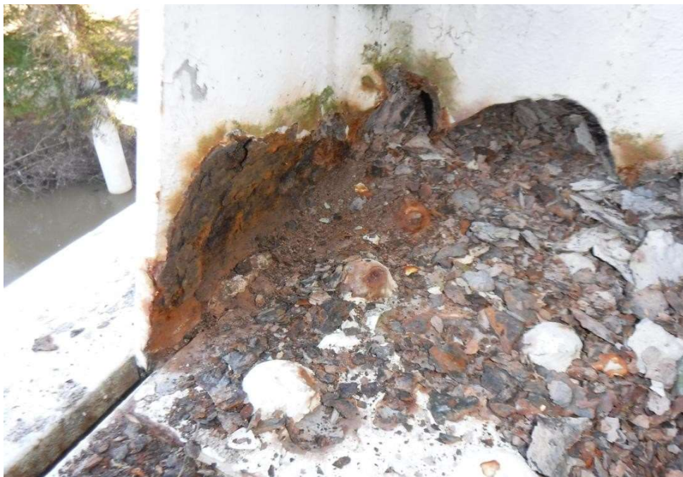
Photo 64 - Lower chord gusset plate condition at Joint L2, Truss 2, Span 5
