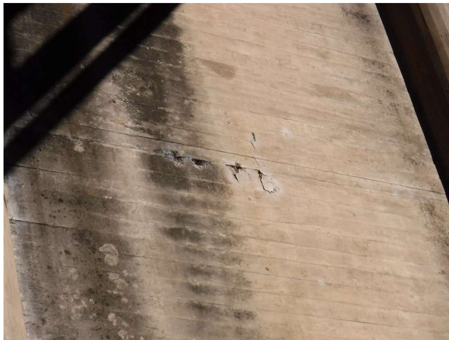
Photo 54 - Localized Delamination and Spalling at Construction Joint on West Face of Pier 6
