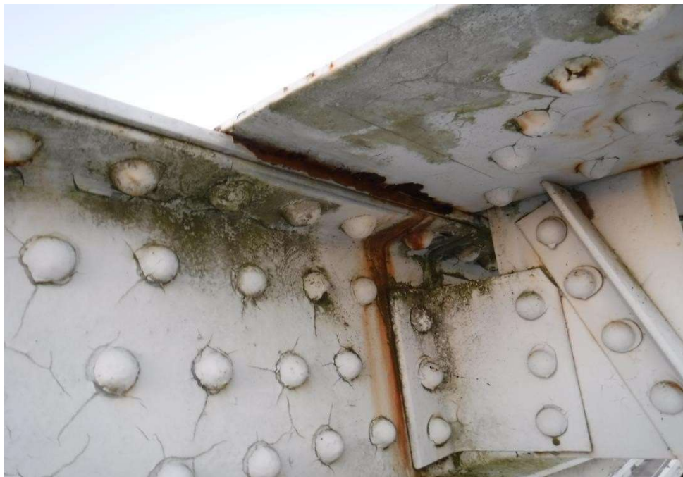
Photo 80 - Upper chord gusset plate condition at Joint U5, Truss 2, Span 6
