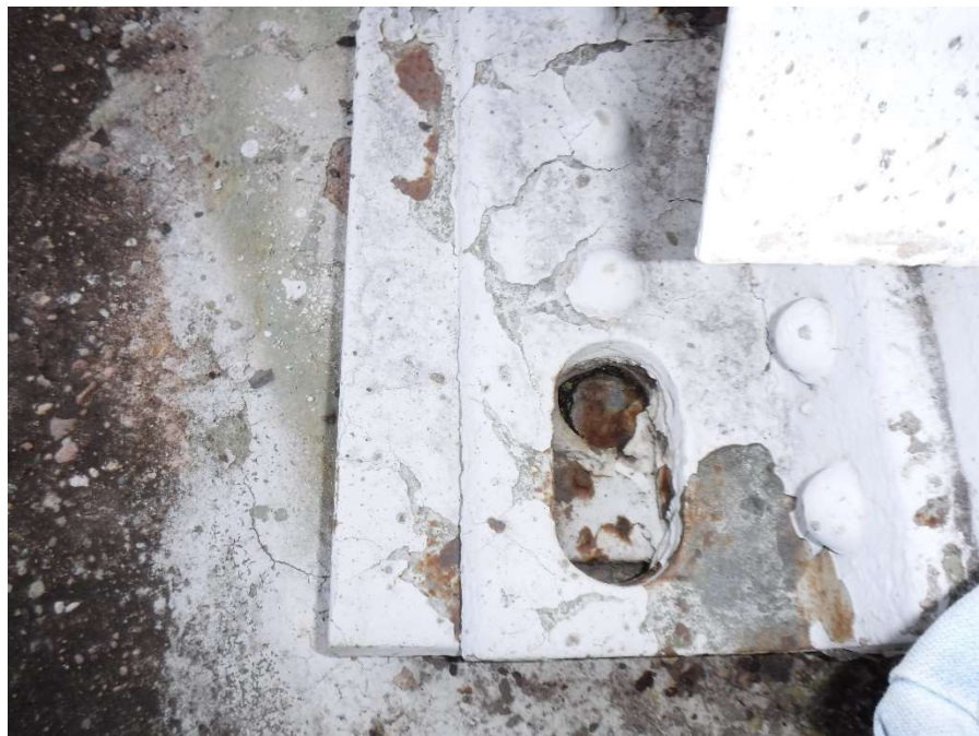
Photo 52 - Failed Anchor Bolt at Joint L9, Truss 2, Span 6
