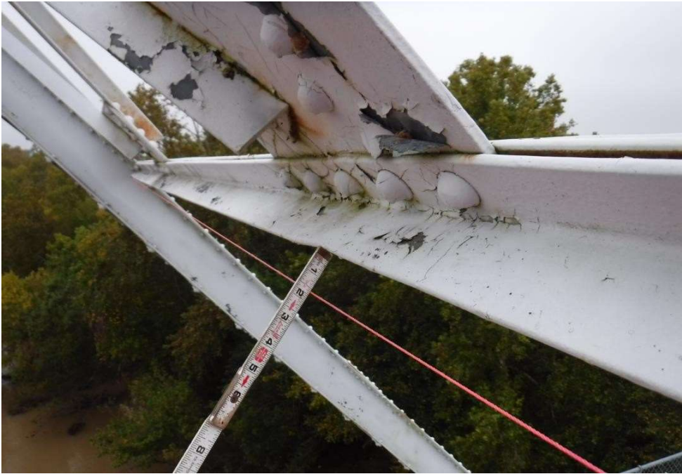
Photo 98 - Cross frame lower chord deformation at Joint U8, Span 5
