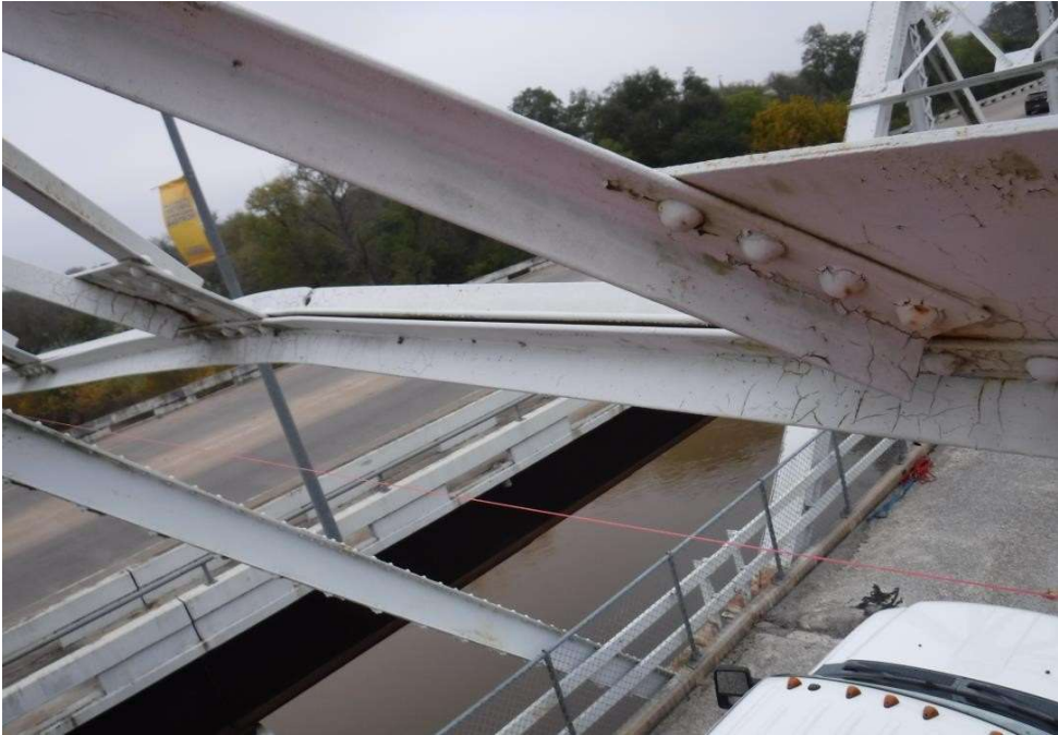
Photo 99 - Cross frame lower chord deformation at Joint U1, Span 6
