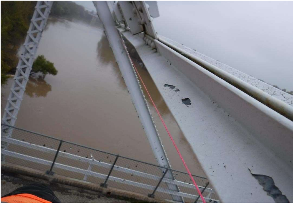
Photo 96 - Cross frame lower chord deformation at Joint U8, Span 4
