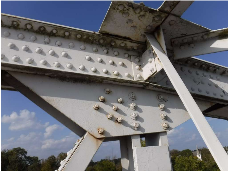
Photo 30 - Repaired Connection to Diagonal and Vertical Members at Joint U6, Truss 2, Span 5
