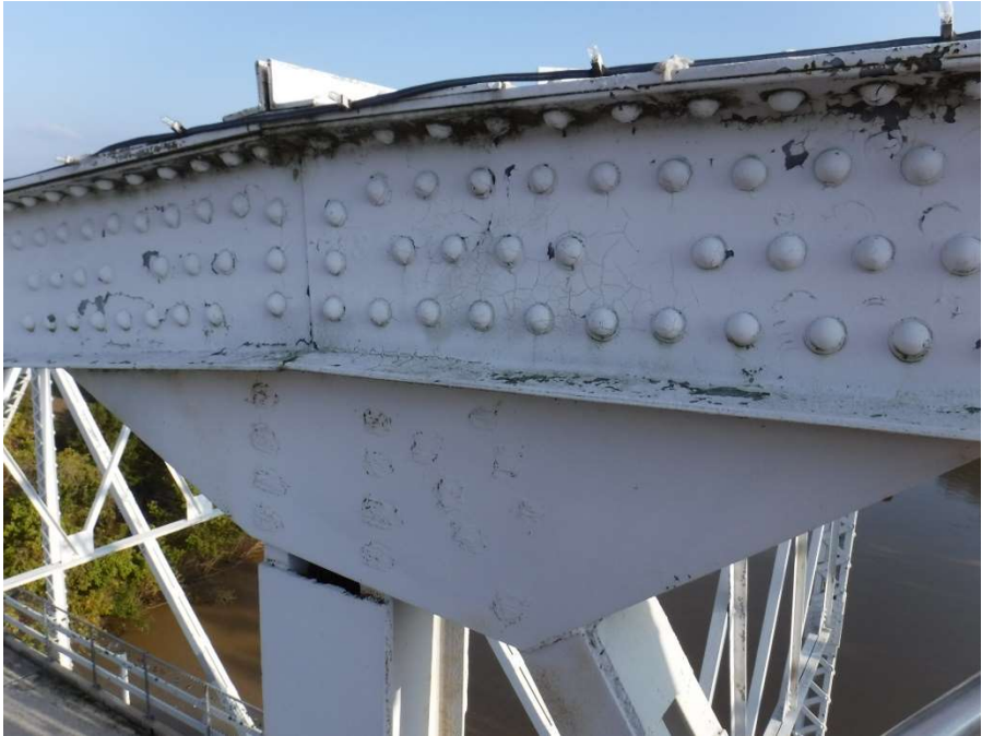
Photo 29 - Repaired Connection to Diagonal and Vertical Members at Joint U6, Truss 2, Span 4
