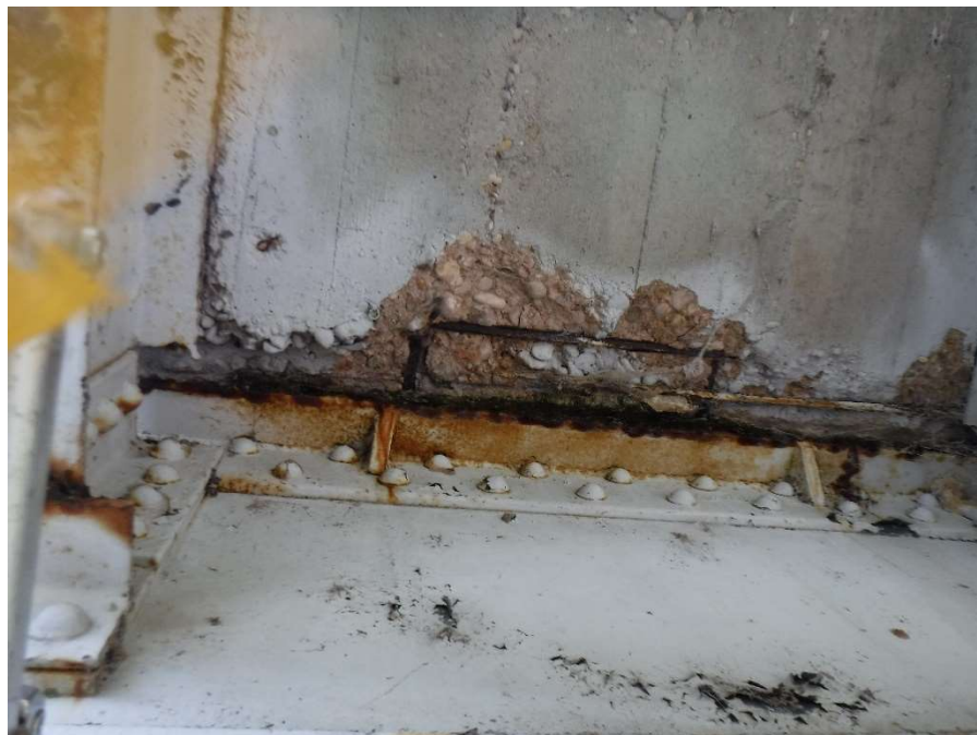
Photo 22 - Typical Spalling on Deck over Floorbeams
