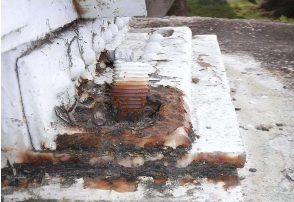
Photo 109 - Exterior anchor bolt condition, missing fastener, missing bolt, at Joint L9, Truss 2, Span 6
