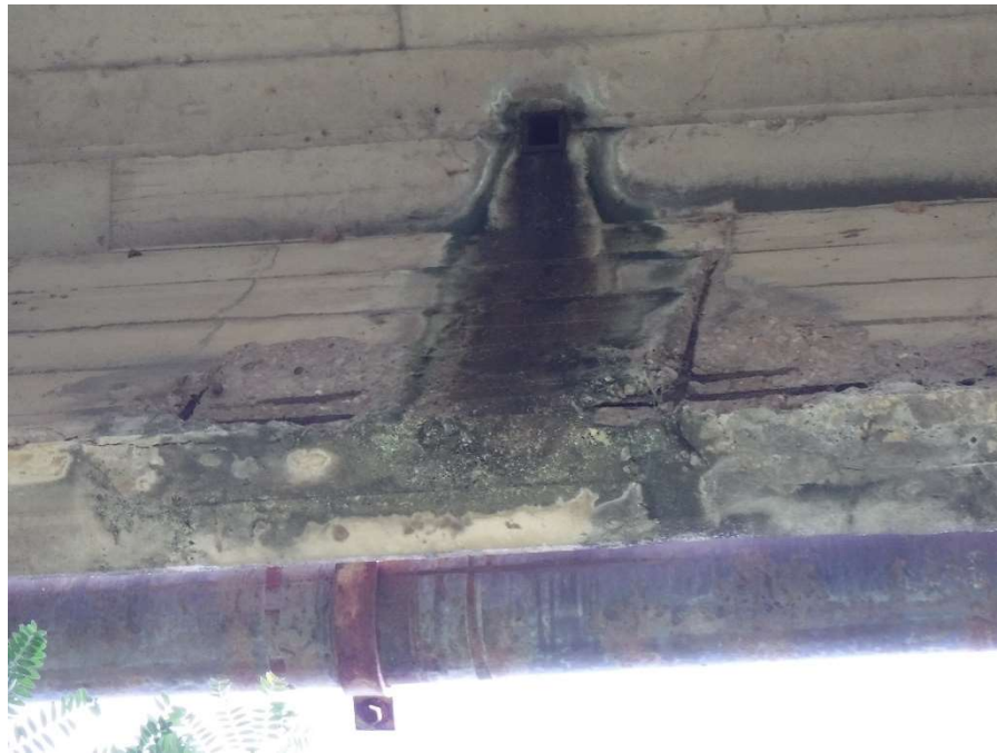
Photo 17 - Transverse Cracking and Cover Spalling on Inside Face of T-beam 1 at Span 13 Drain
