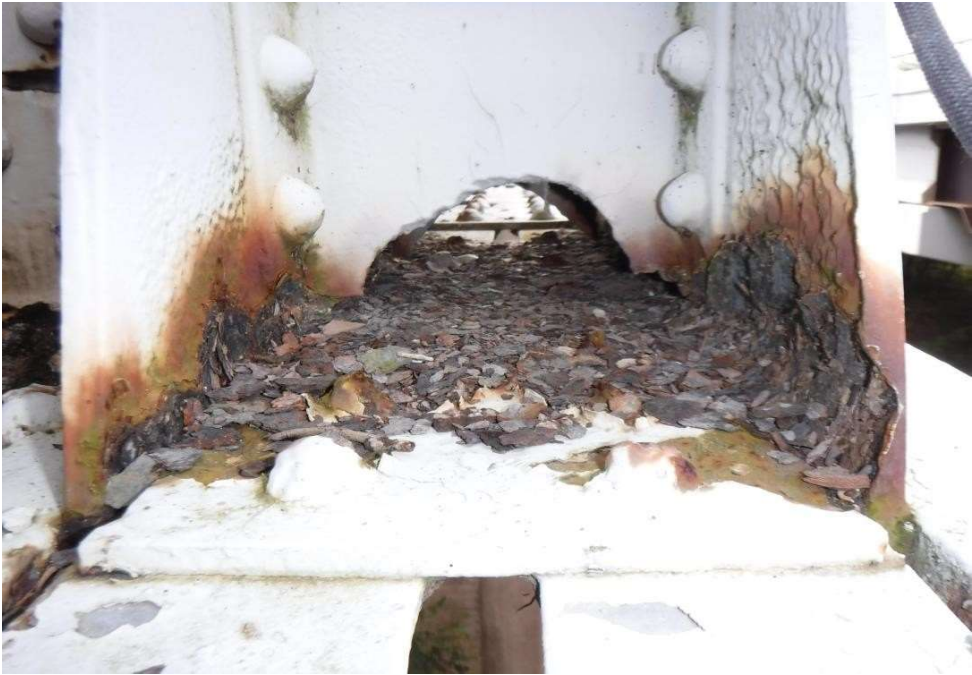
Photo 76 - Lower chord gusset plate condition at Joint L7, Truss 2, Span 6
