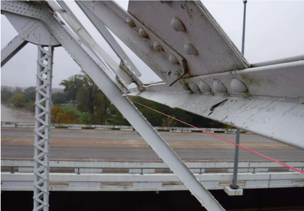
Photo 97 - Cross frame lower chord deformation at Joint U1, Span 5
