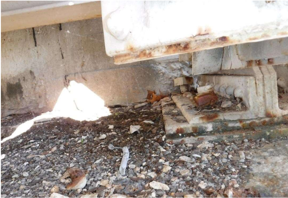
Photo 102 – Interior anchor bolt condition at Joint L0, Truss 1, Span 4
