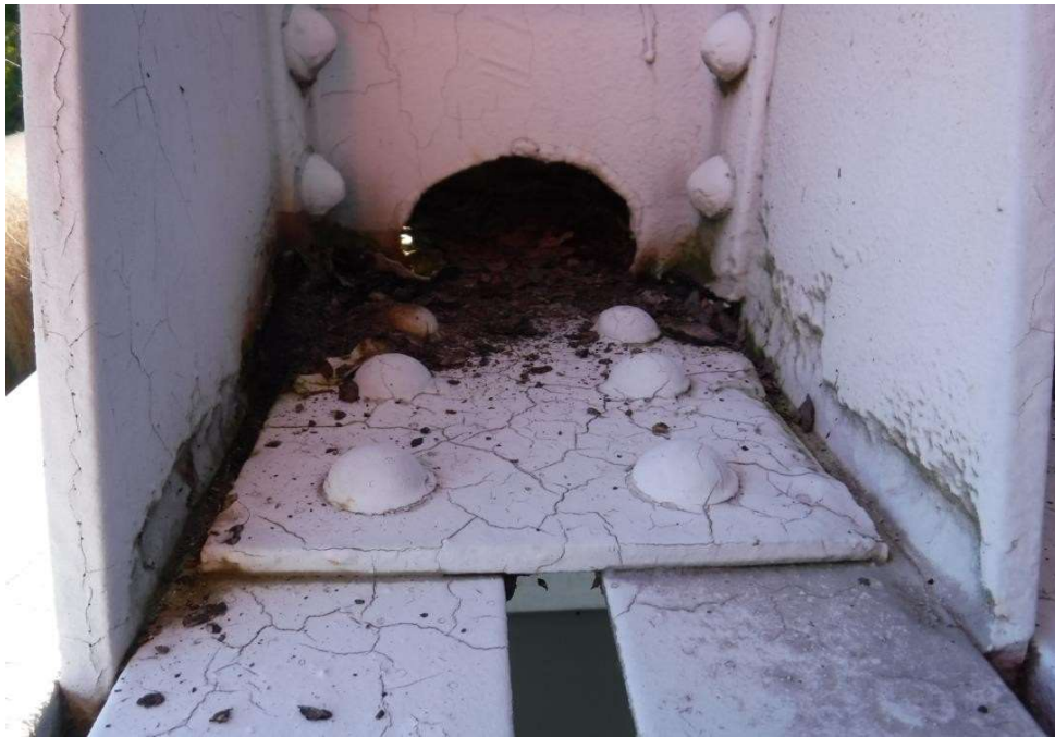
Photo 63 - Lower chord gusset plate condition at Joint L6, Truss 1, Span 5
