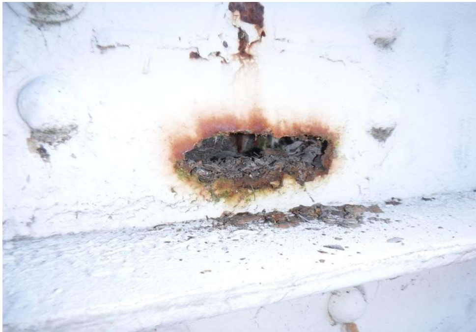
Photo 65 - Lower chord gusset plate condition at Joint L5, Truss 2, Span 5
