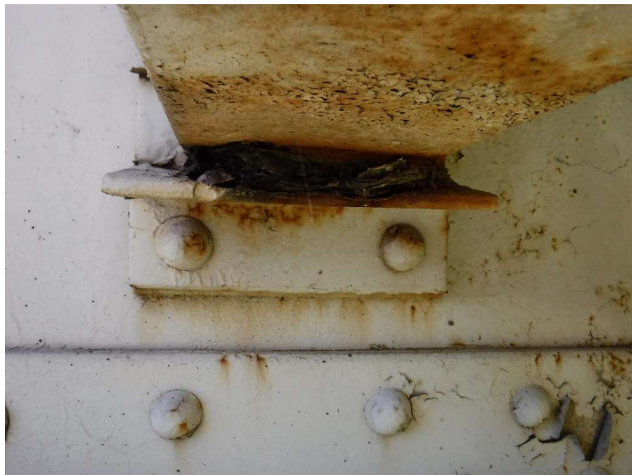
Photo 50 - Typical Pack Rust Condition at Exterior Stringer Bearing Seat
