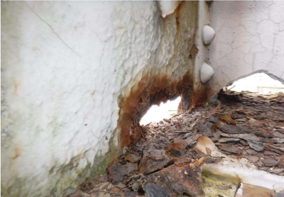
Photo 75 - Lower chord gusset plate condition at Joint L6, Truss 2, Span 6
