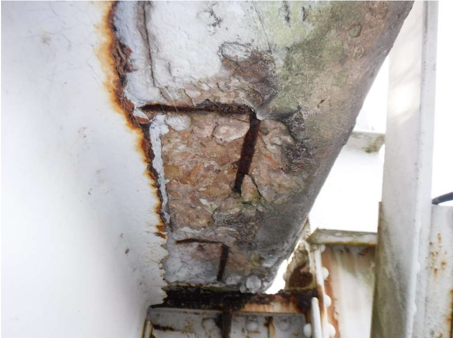
Photo 23 - Typical Spalling on Deck Overhang Near Joint
