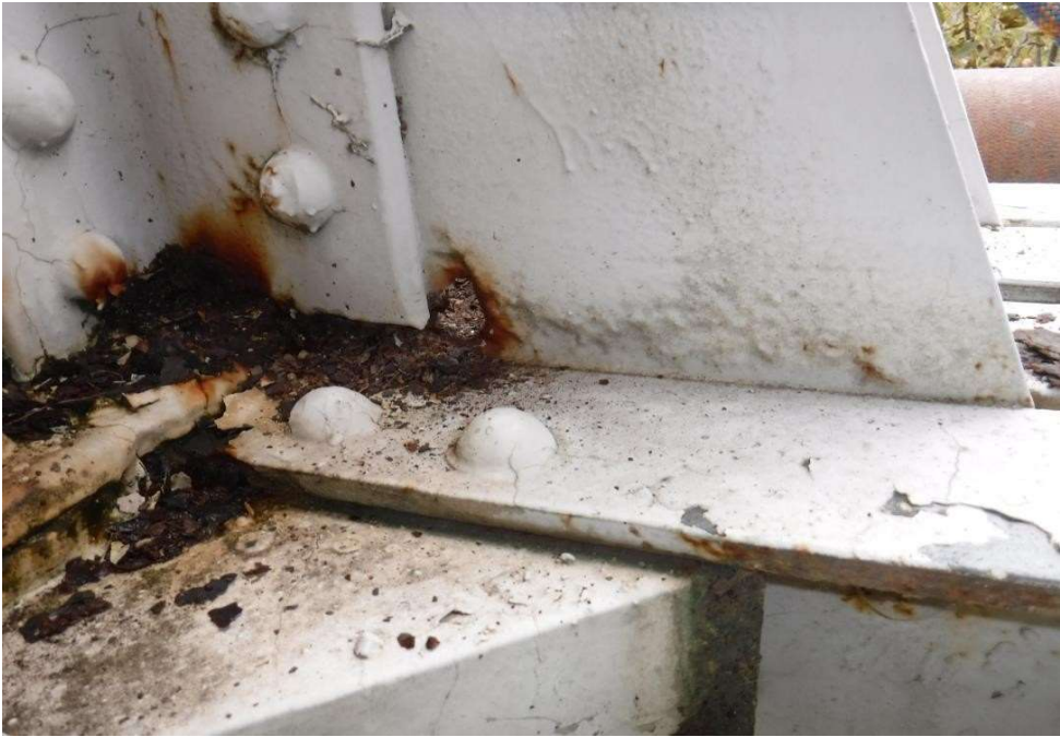
Photo 68 - Lower chord gusset plate condition at Joint L3, Truss 1, Span 6
