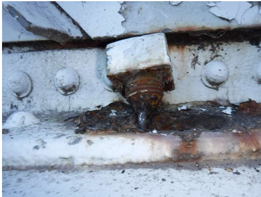
Photo 51 - Section Loss on Exterior Anchor Bolt at Joint L9, Truss 2, Span 5
