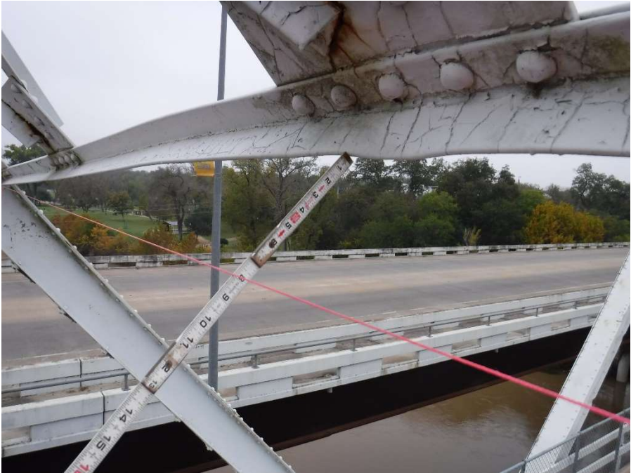
Photo 31 - Impact Deformation up to 8 inches at Lower Chord of Cross Frame at U8 in Span 6
