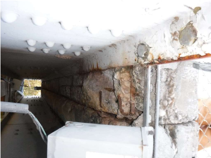
Photo 24 - Cover Spalling on Deck Soffit along Joint at Bent 6
