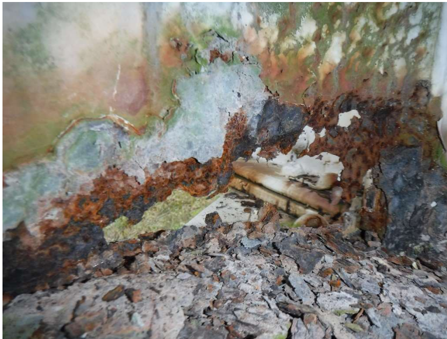
Photo 45 - Full Thickness 6"x3" Section Loss on Interior Gusset Plate at Joint L3, Truss 2, Span 6
