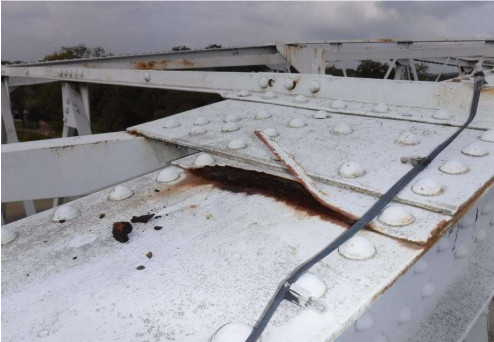
Photo 83 - Upper chord filler plate condition at Joint U7, Truss 1, Span 5
