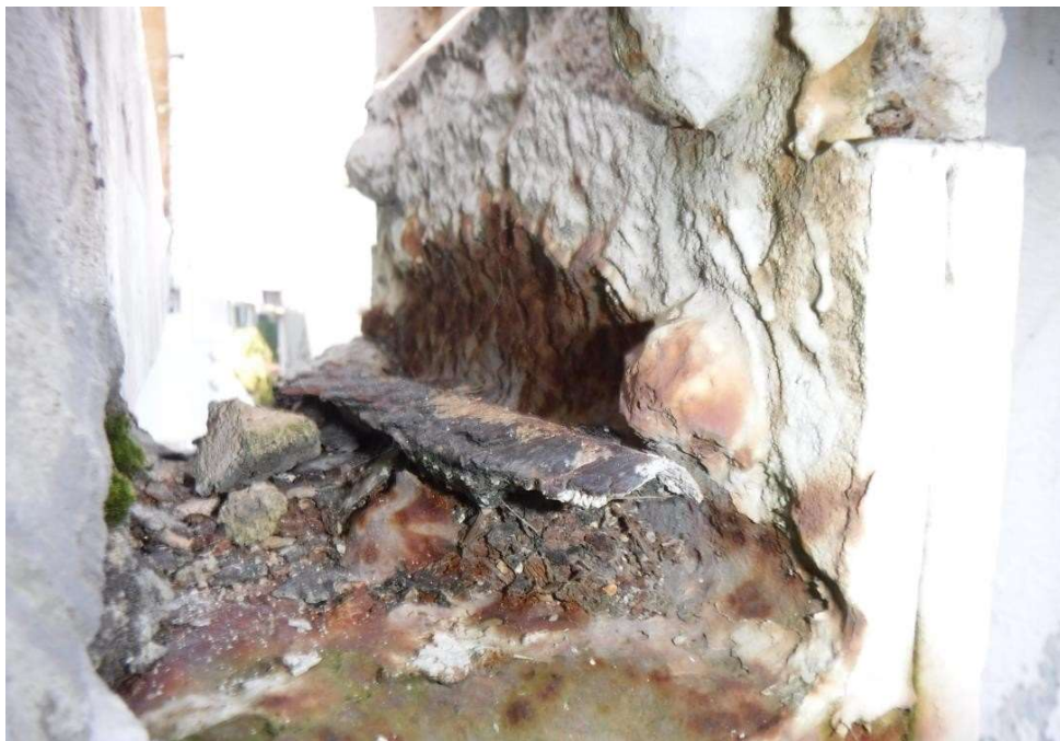
Photo 92 - Floorbeam to vertical connection angle condition at Joint L6, Truss 2, Span 5
