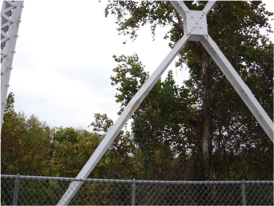
Photo 40 - Torsional Deformation on Member L5U4, Truss 1, Span 6
