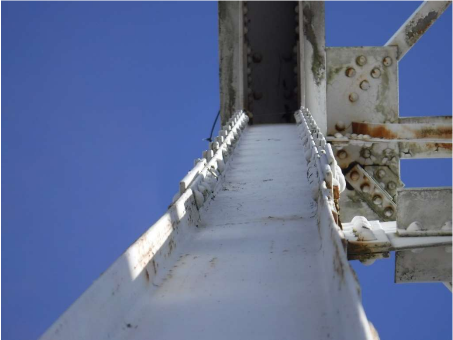
Photo 39 - Butt Weld Joint at Repaired Member L4U4, Truss 2, Span 4
