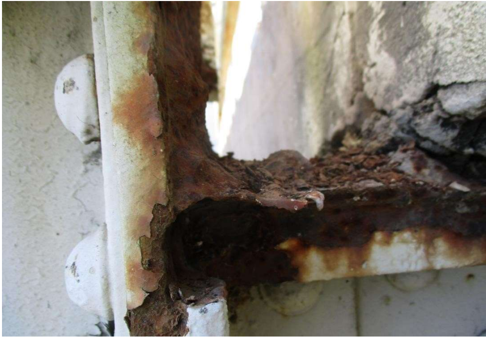
Photo 88 - Floorbeam to vertical connection angle condition at Joint L6, Truss 2, Span 4
