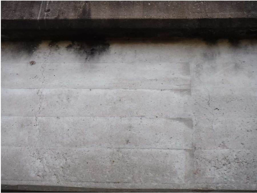
Photo 16 - Transverse Cracking on Stem of T-beam 4 at Span 21
