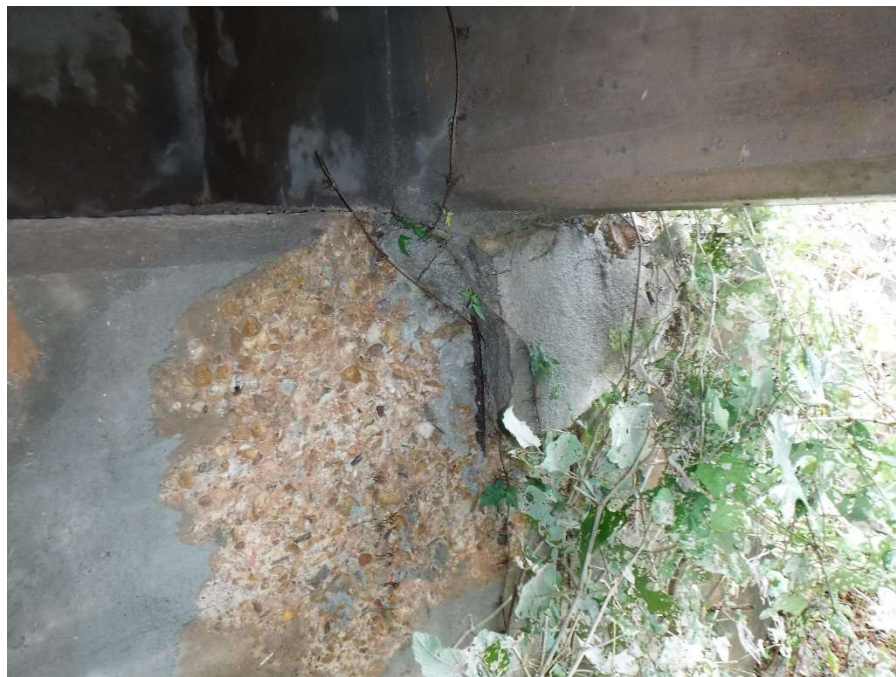
Photo 18 - Cover Spalling on West Abutment Cap
