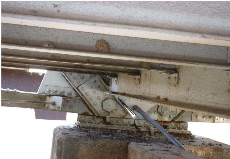
Photo 107 - Interior anchor bolt condition at Joint L9, Truss 2, Span 5
