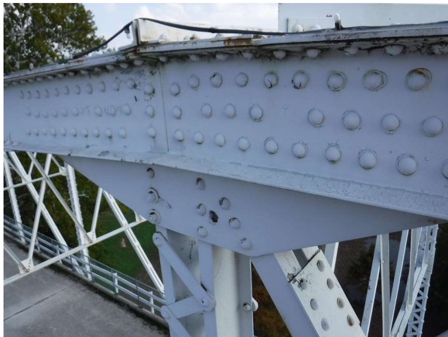
Photo 28 - Torch Hole and 1/4" Deep Gouge on Exterior Gusset Plate at Joint U5, Truss 2, Span 4
