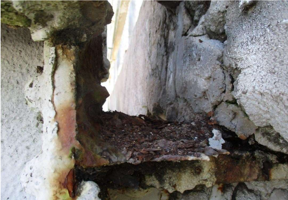
Photo 89 - Floorbeam to vertical connection angle condition at Joint L7, Truss 2, Span 4
