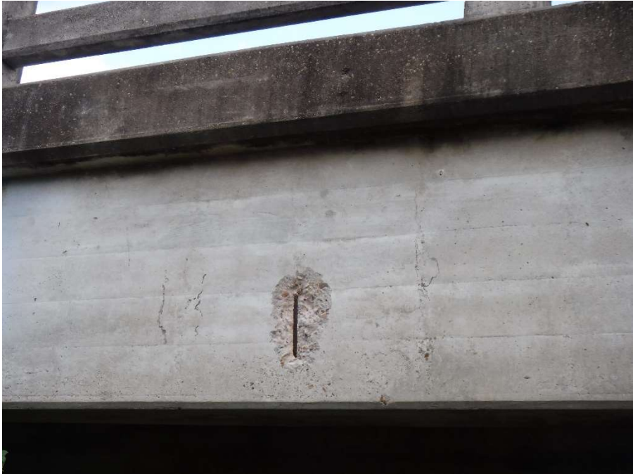
Photo 15 - Delamination and Cover Spalling on Stem of T-beam 4 at Span 21
