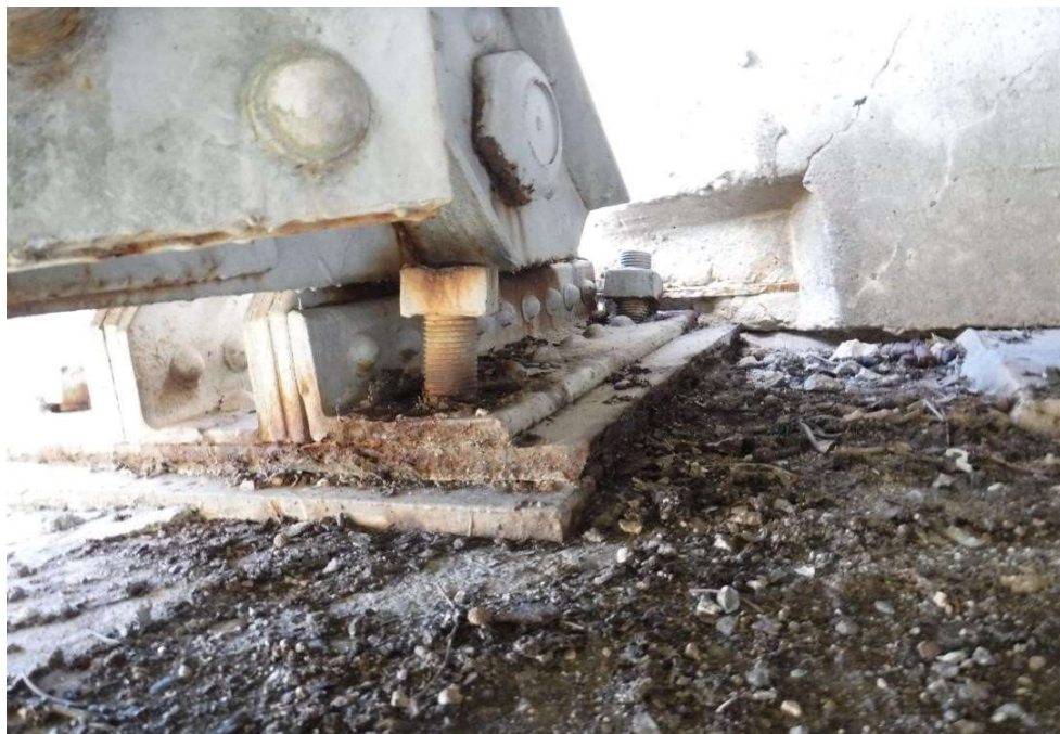
Photo 108 - Interior anchor bolt condition at Joint L9, Truss 1, Span 6
