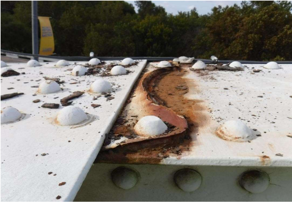
Photo 86 - Upper chord filler plate condition at Joint U8, Truss 2, Span 6
