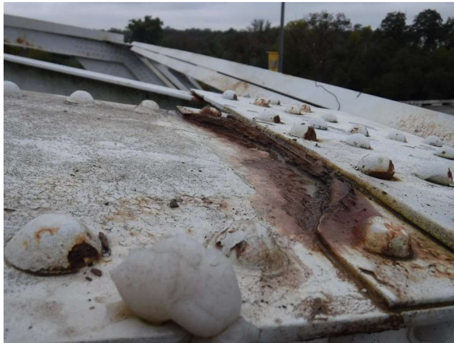
Photo 25 - Typical Condition of Filler Plate and Upper Chord Cover Plate at Joints U1 and U8
