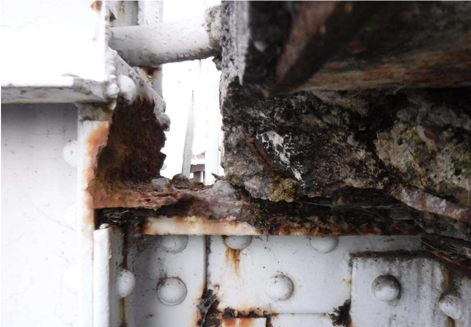
Photo 93 - Floorbeam to vertical connection angle condition at Joint L2, Truss 2, Span 6
