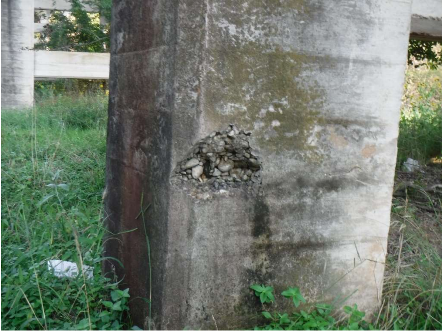
Photo 20 - Unconsolidated Concrete Spalling on Column at Bent 14
