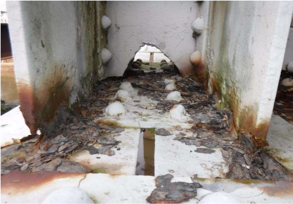
Photo 74 - Lower chord gusset plate condition at Joint L5, Truss 2, Span 6
