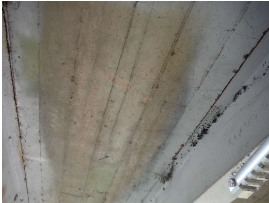
Photo 21 - Typical Cracking on Deck Soffit at Main Spans
