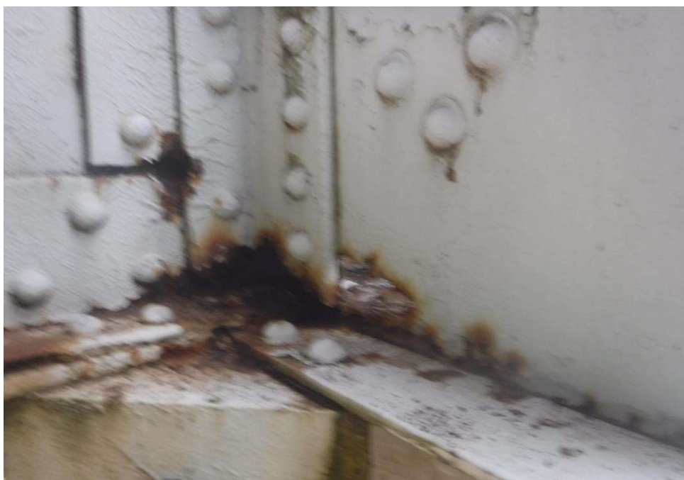
Photo 58 - Lower chord gusset plate condition at Joint L3, Truss 2, Span 4
