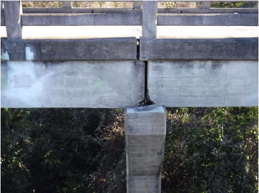
Photo 14 - Cover spalling at T-beam 4 over Bent 8
