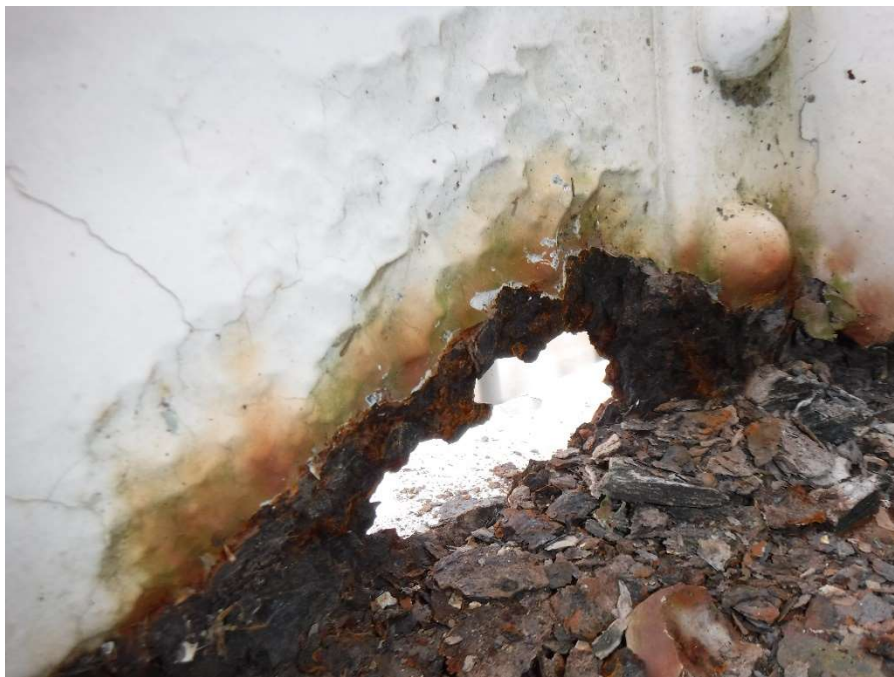
Photo 46 - Full Thickness 3"x2" Section Loss on Exterior Gusset Plate at Joint L3, Truss 2, Span 6
