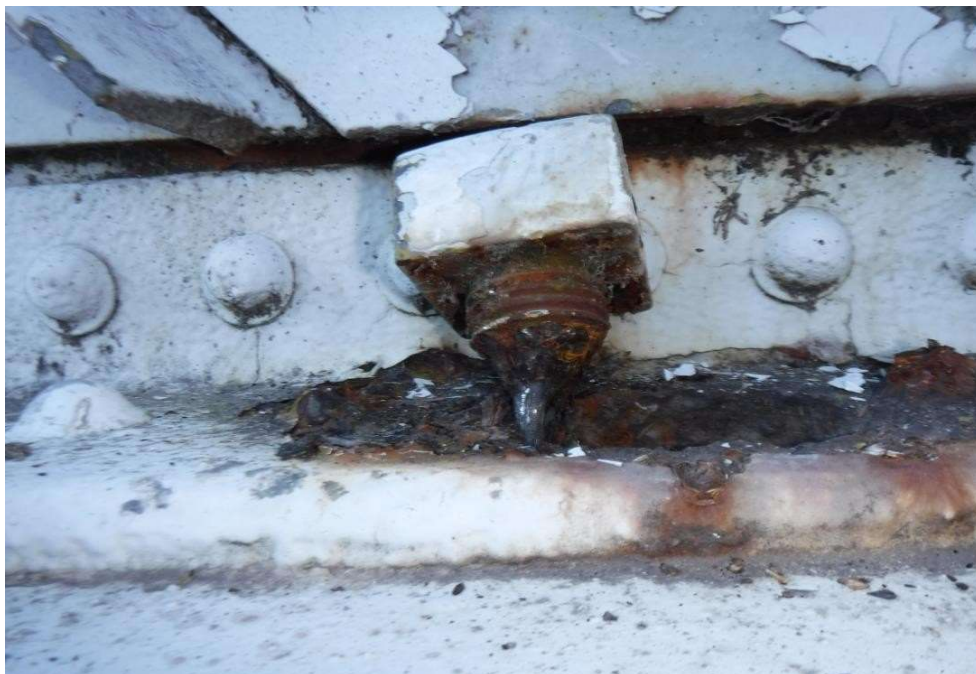
Photo 106 - Exterior anchor bolt condition at Joint L9, Truss 2, Span 5
