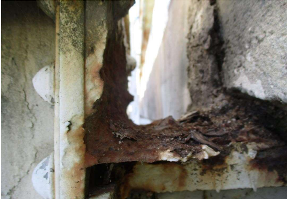
Photo 87 - Floorbeam to vertical connection angle condition at Joint L5, Truss 2, Span 4
