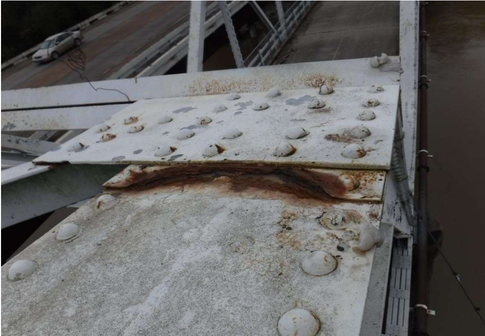
Photo 85 - Upper chord filler plate condition at Joint U1, Truss 1, Span 6
