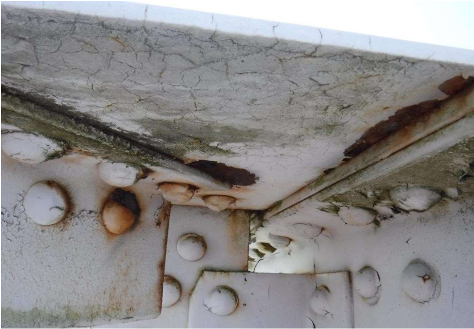
Photo 78 - Upper chord gusset plate condition at Joint U5, Truss 1, Span 4
