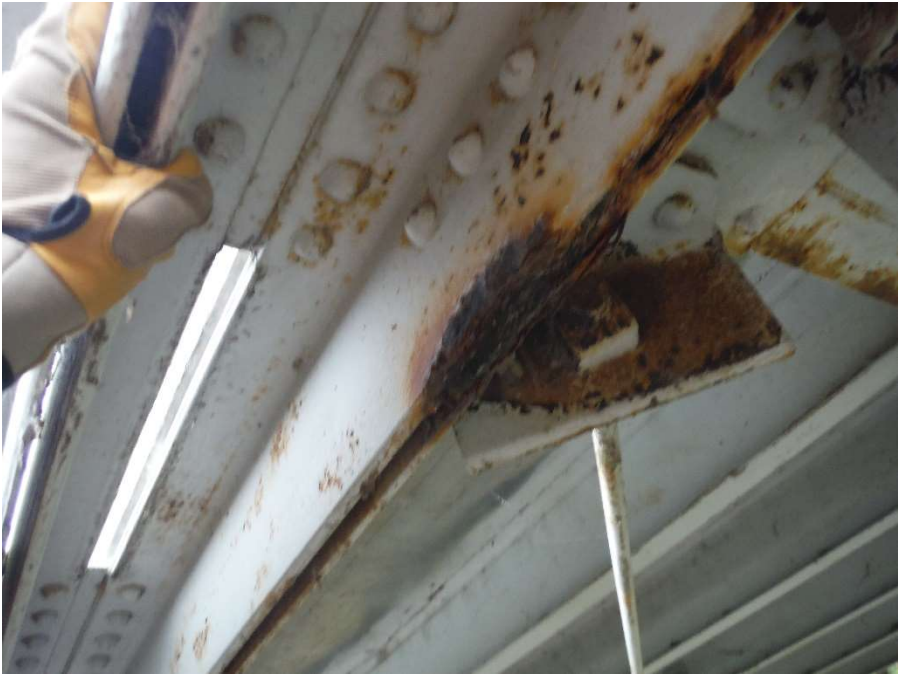
Photo 42 - Typical Pack Rust, Corrosion, and Section Loss on Lower Chord
