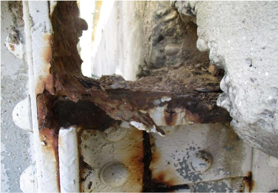
Photo 90 - Floorbeam to vertical connection angle condition at Joint L8, Truss 2, Span 4
