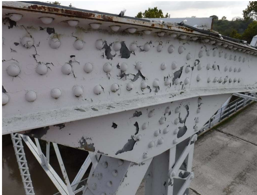
Photo 33 - Typical Paint Failure on Truss Members
