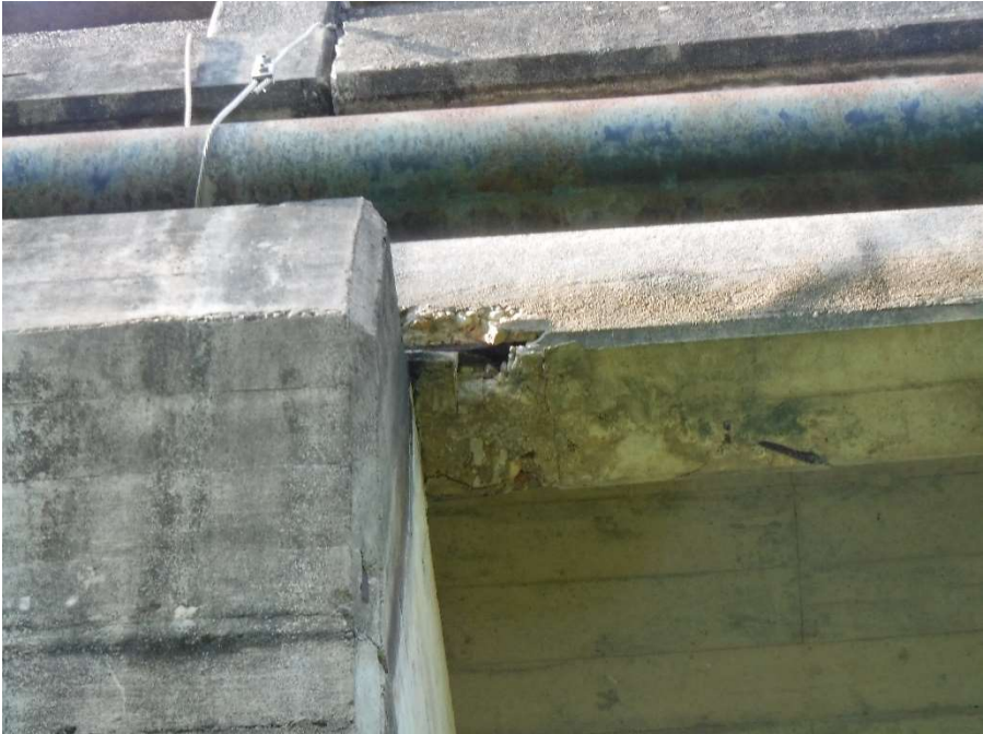
Photo 13 - Cover Spalling on T-beam 1 over Bent 14
