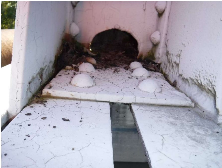
Photo 43 - Typical Gusset Plate Section Loss at Joints L2 through L7 in all Trusses
