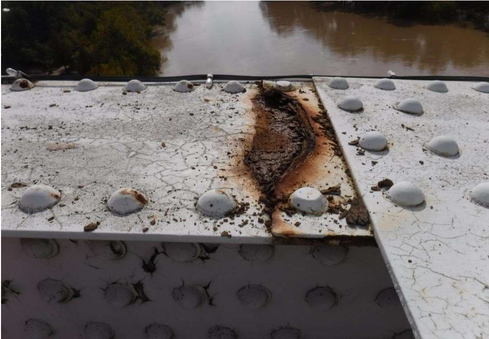
Photo 81 - Upper chord filler plate condition at Joint U8, Truss 1, Span 4
