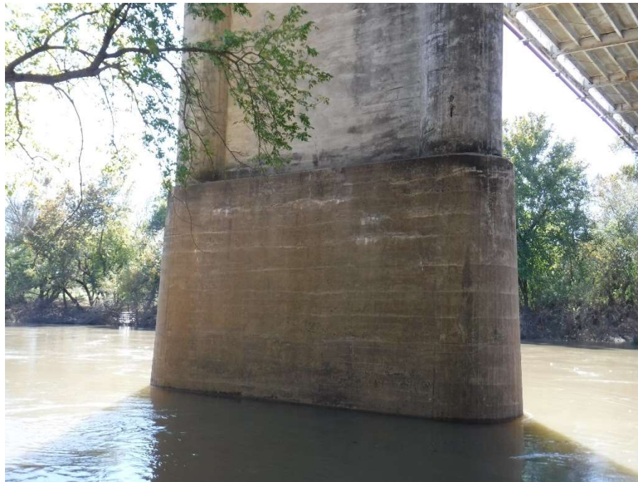
Photo 53 - Horizontal Cracking and Efflorescence on East Face of Pier 5
