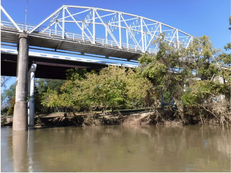
Photo 117 – Erosion of east channel bank through Chestnut St. bridges
