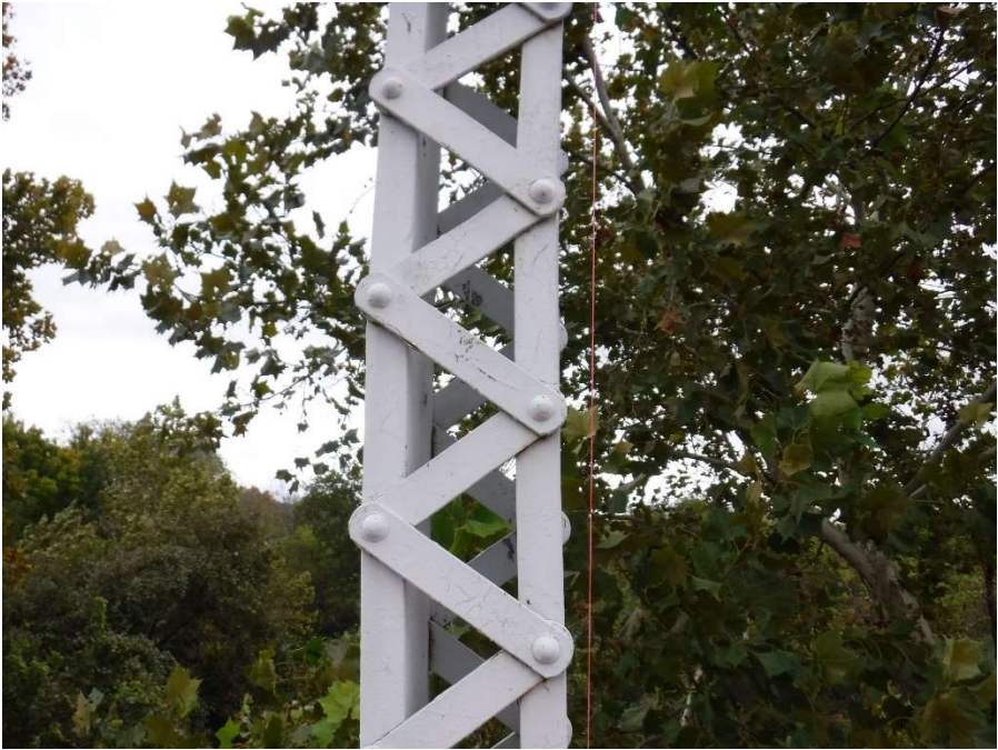
Photo 36 - 2-1/2" Deflection of Vertical Member L2U2, Truss 1, Span 6
