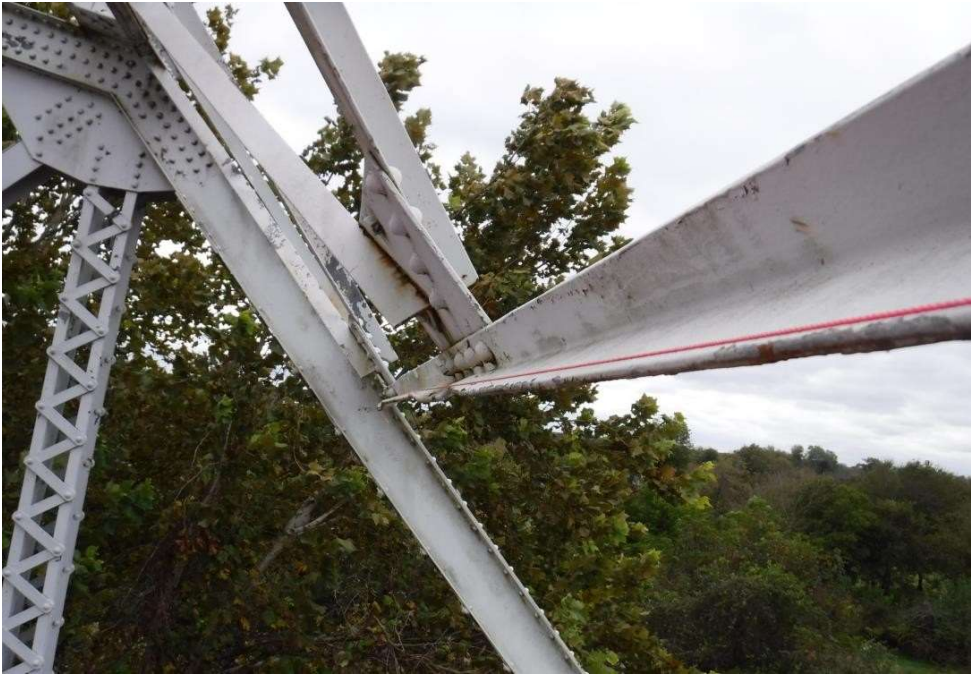
Photo 100 - Cross frame lower chord deformation at Joint U8, Span 6
