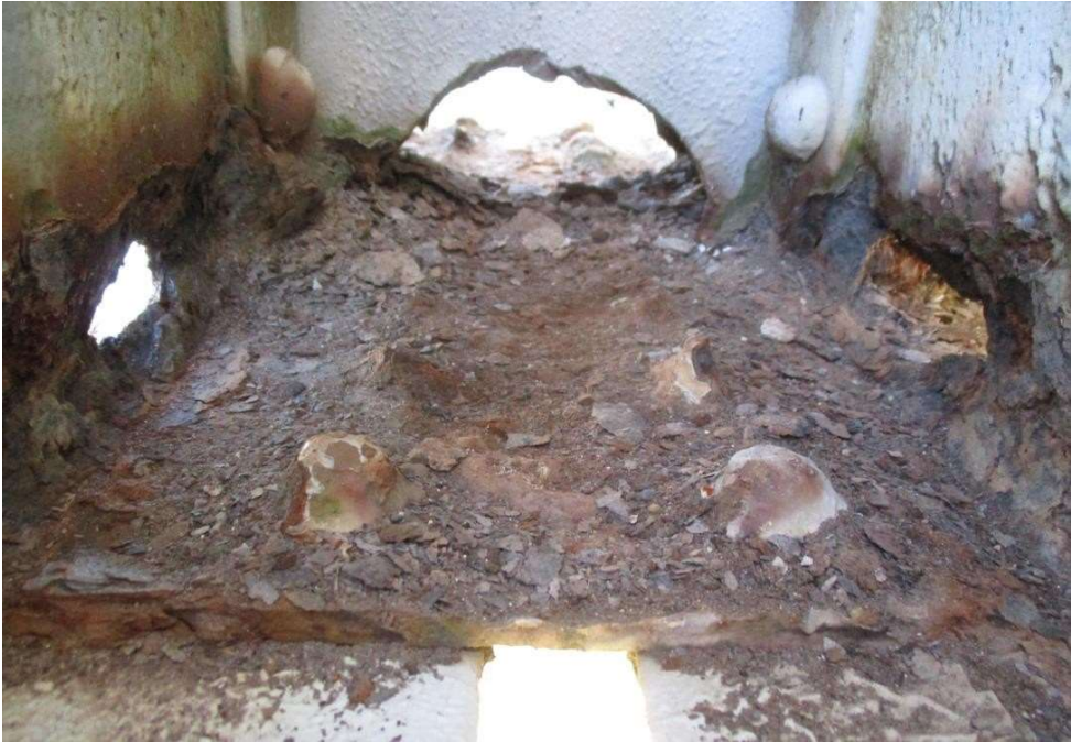
Photo 61 - Lower chord gusset plate condition at Joint L6, Truss 2, Span 4
