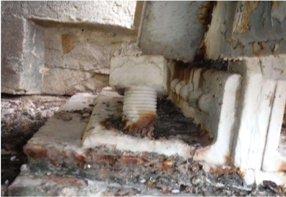
Photo 110 - Interior anchor bolt condition at Joint L9, Truss 2, Span 6
