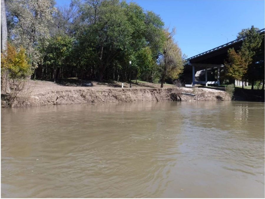
Photo 118 – Erosion of east channel bank upstream of Chestnut St. bridges
