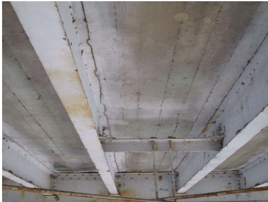
Photo 49 - Typical Section Loss along Stringer Top Flanges
