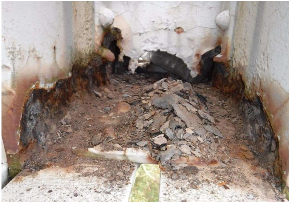
Photo 69 - Lower chord gusset plate condition at Joint L4, Truss 1, Span 6
