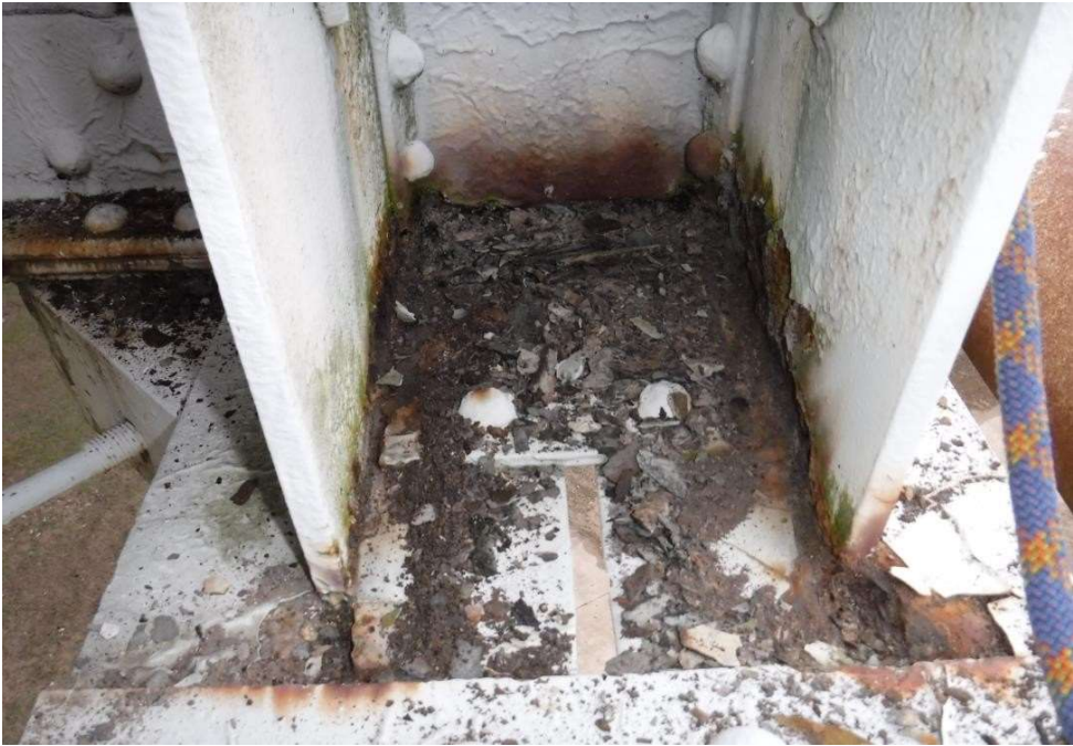
Photo 56 - Lower chord gusset plate condition at Joint L5, Truss 1, Span 4
