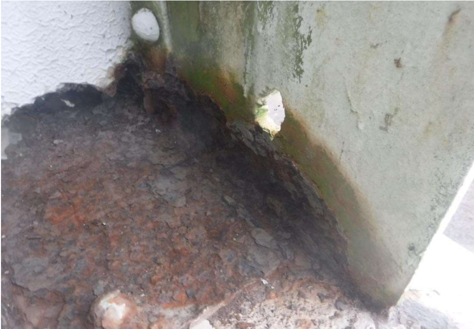
Photo 59 - Lower chord gusset plate condition at Joint L4, Truss 2, Span 4
