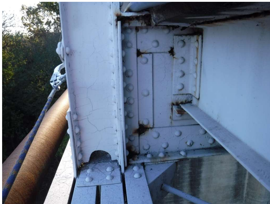
Photo 48 - Typical Localized Pack Rust at Ends of Interior Floorbeam
