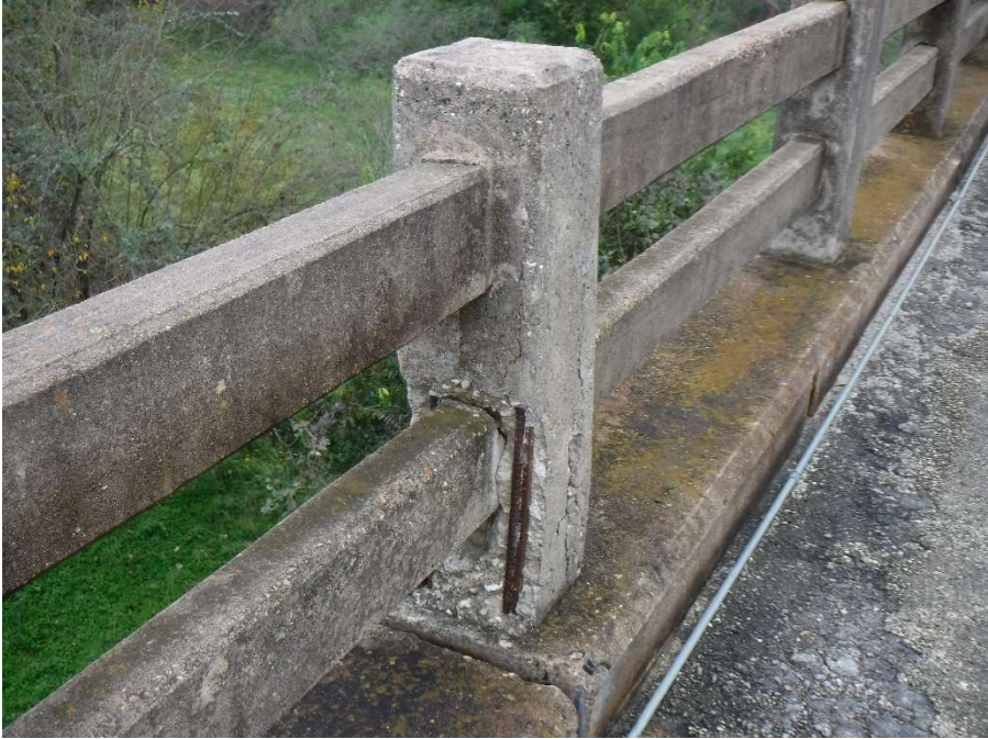
Photo 12 - Delamination and Cover Spalling at South Rail Post over Bent 13
