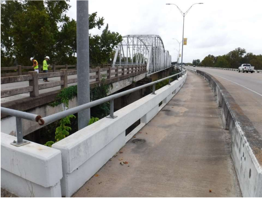
Photo 2 - East Approach Bridge Elevation
