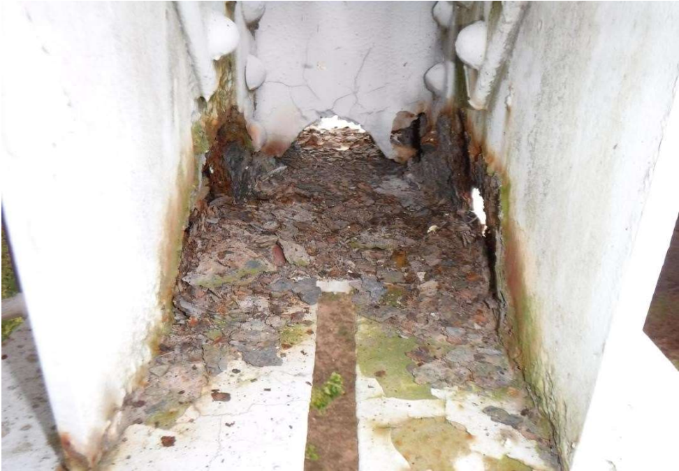
Photo 71 - Lower chord gusset plate condition at Joint L3, Truss 2, Span 6
