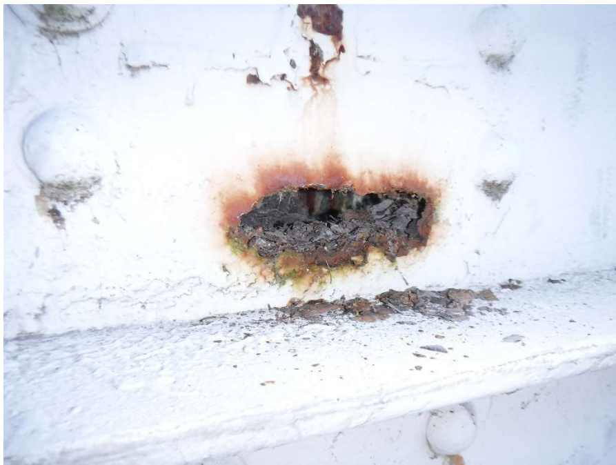
Photo 44 - Full Thickness 1"x4" Section Loss on Exterior Gusset Plate at Joint L5, Truss 2, Span 5
