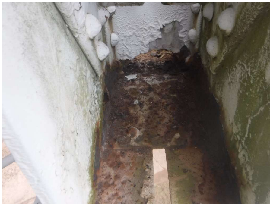
Photo 34 - Typical Condition of Lower Chord Channels
