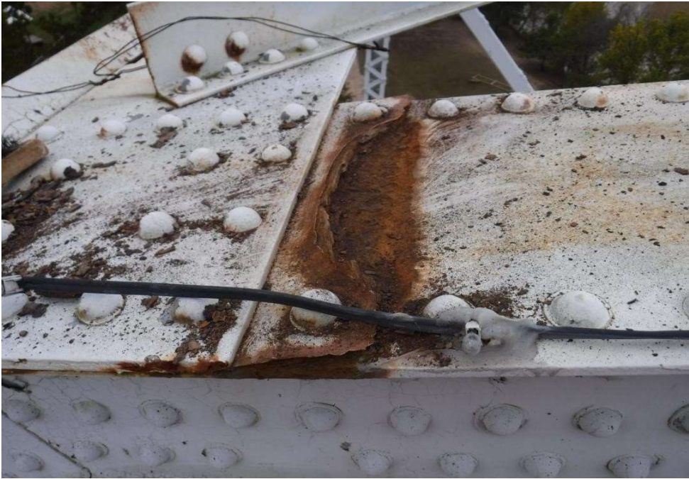
Photo 82 - Upper chord filler plate condition at Joint U1, Truss 2, Span 4
