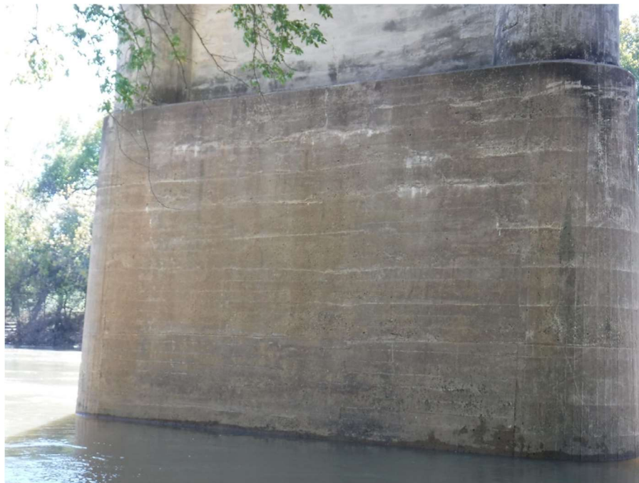
Photo 116 – General condition of concrete bents above water. Heavier abrasion below water level.
