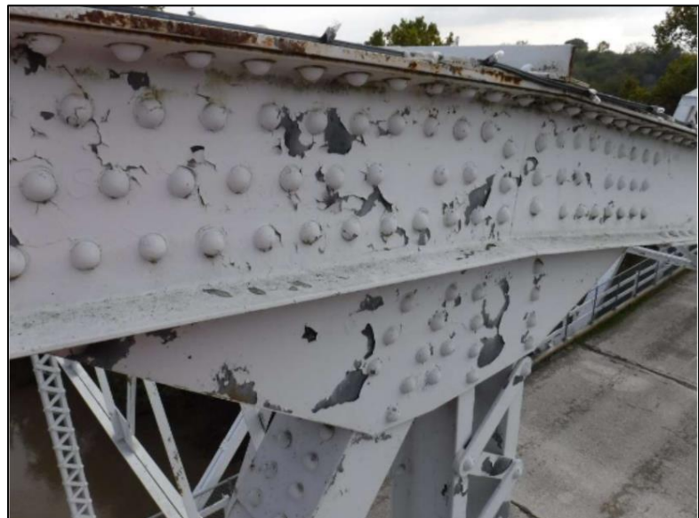
Figure 7: Failing Lead Paint on the Old Iron Bridge
